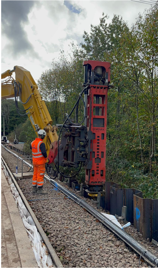
Figure 2: A close up view of the Movax attachment re-driving piles with it's DH25 impact hammer
